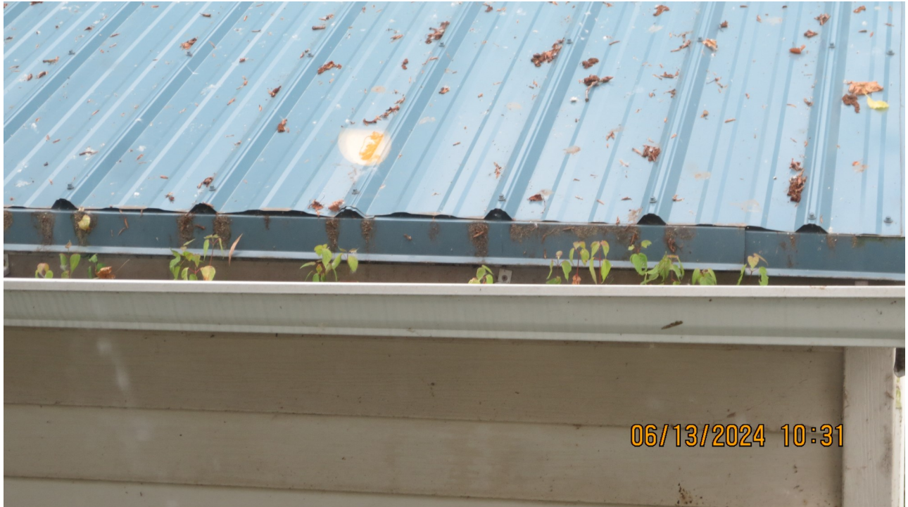
Image #3 showing poor maintenance of encroachment.
