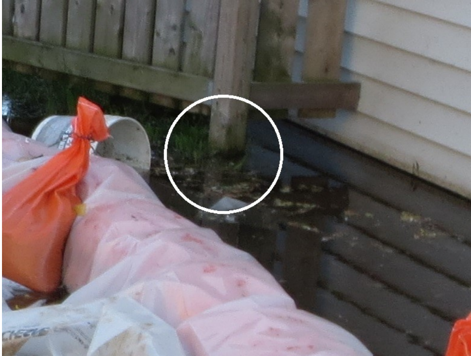
Image #17. Close-up of damage to fence post.
