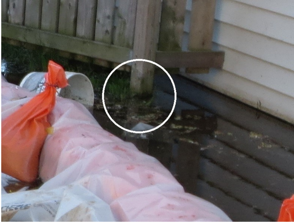
Image #3 close-up view of fence deterioration and rotting in 2019.
