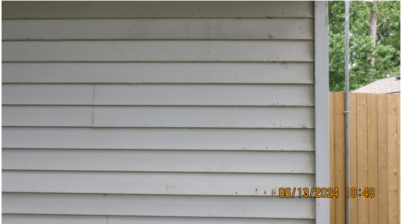
Image #1 showing poor maintenance of encroachment.
