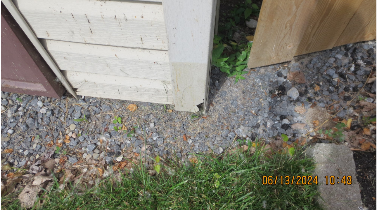
Image #4 showing poor maintenance of encroachment.
