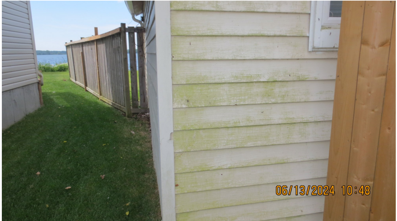
Image #2 showing poor maintenance of encroachment.
